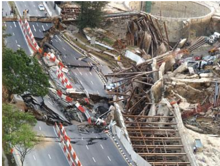
Fig.1.1 Singapore Nicoll Highway collapse adjacent to an excavation
